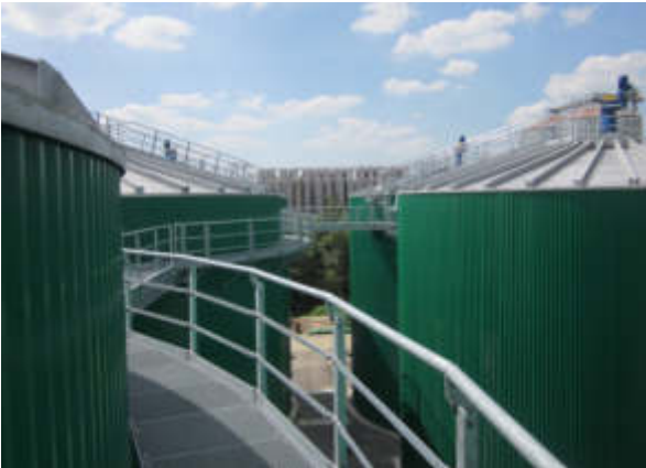
Biogasanlage Dorsten 8 Fermenter mit jeweils 3.200m 3 Biogas plant in Dorsten 8 fermenters, each with a capacity of 3,200 m 3 .
